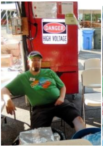
Not sure why but Pete Skinder is leaning against The High Voltage power panel in a Water booth!
